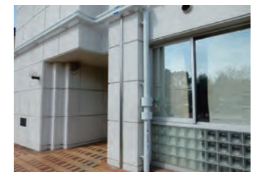
Aboveground water piping
